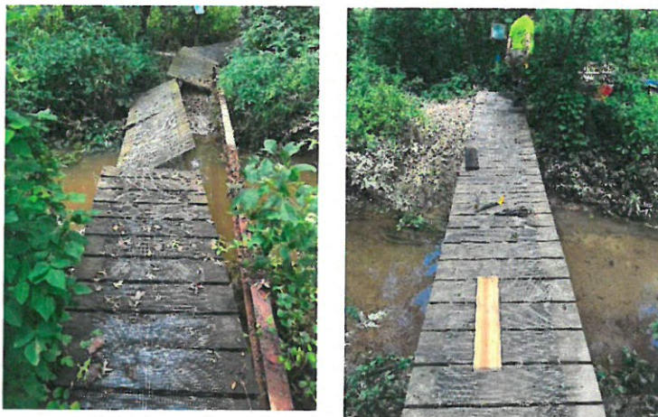
Figure 2: Flooding Damage from 4 inches of rain
