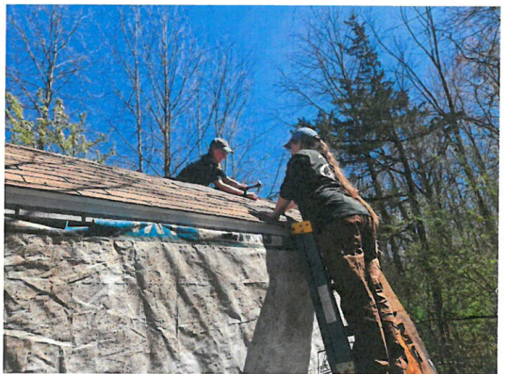
Ginger and Sandra putting the finishing touches on the gray shed roof.
