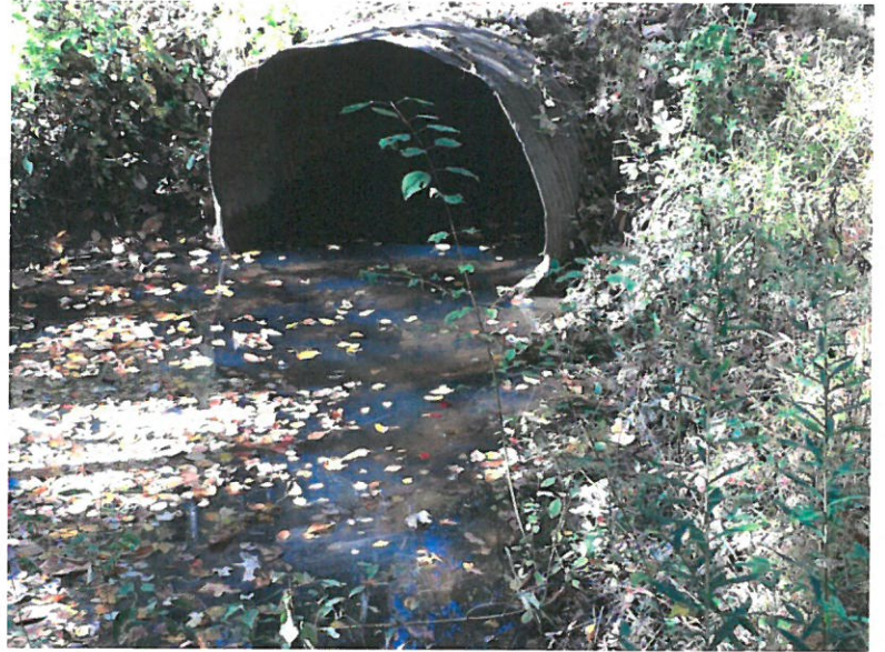
Removal of this culvert will now allow water to flow more naturally along this section of silver Brook, and will reduce scouring caused by the constriction of the pipe.
