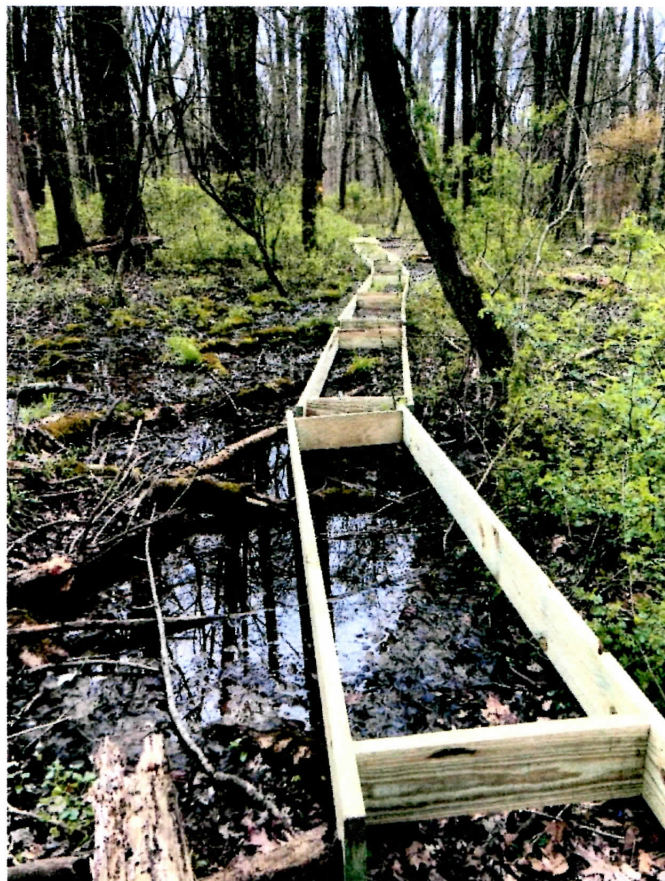
New boardwalk being built along the connector trail by volunteer Steve Gruber
